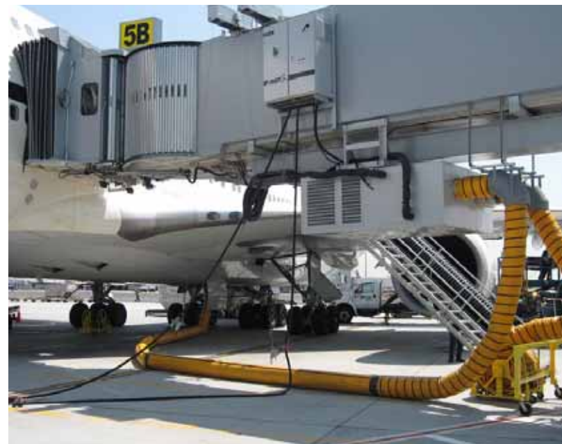
Preconditioned air units (PCAs), like the one pictured above, use 10 times less fuel than a typical 737's onboard auxiliary power unit.
